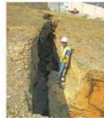
Tension crack at the back of the slide mass
