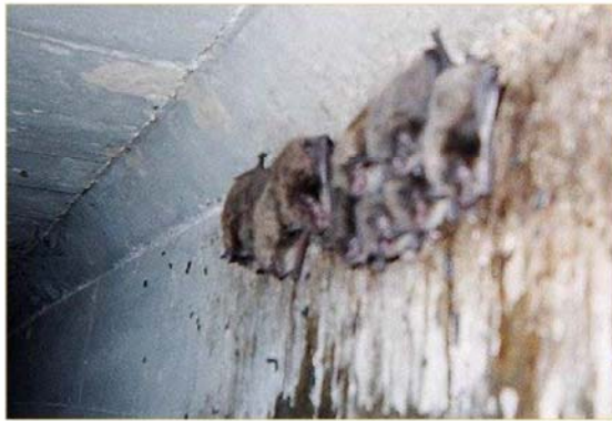
Photo 1: Bats hanging from cracks along support beams
