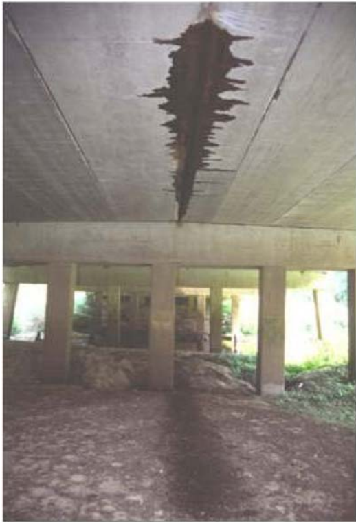
Photo 7: Staining along longitudinal joint.
