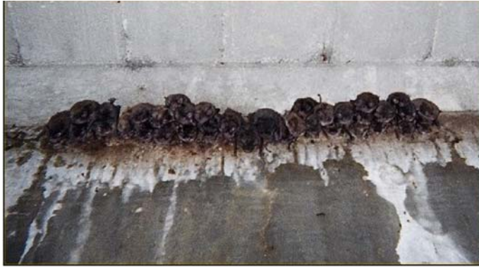
Photo 11: Bats roosting & associated staining
