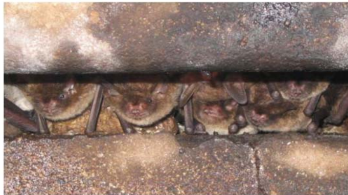
Photo 2: Visible bats within an expansion joint
