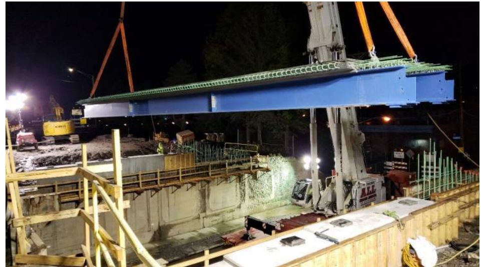
Erection of First Module, Note the Bearings on the New Beam Seats
