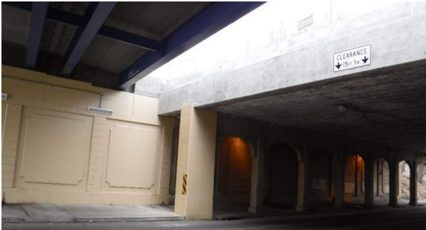
Encasement of Remaining Beam and Pier Column – Note the Railroad Ballast Toe Wall
